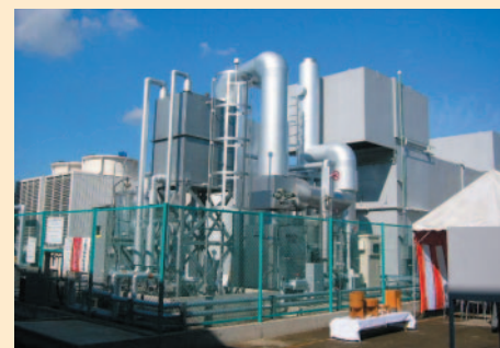
Photo: Natural gas cogeneration system at Oyama Chemical
